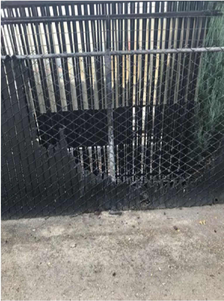
Melted fencing from a fire in Cooper Ct.
