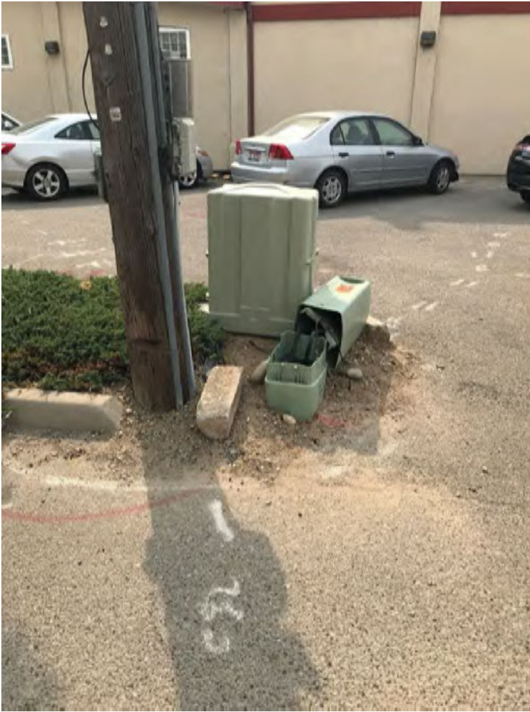
Damaged utility box in alley behind DWF Wholesale Florist.
