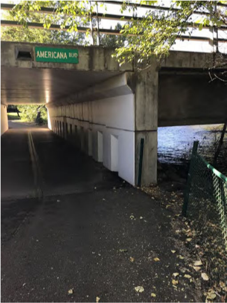
Missing section of fence giving access underneath the Americana Blvd. bridge.
