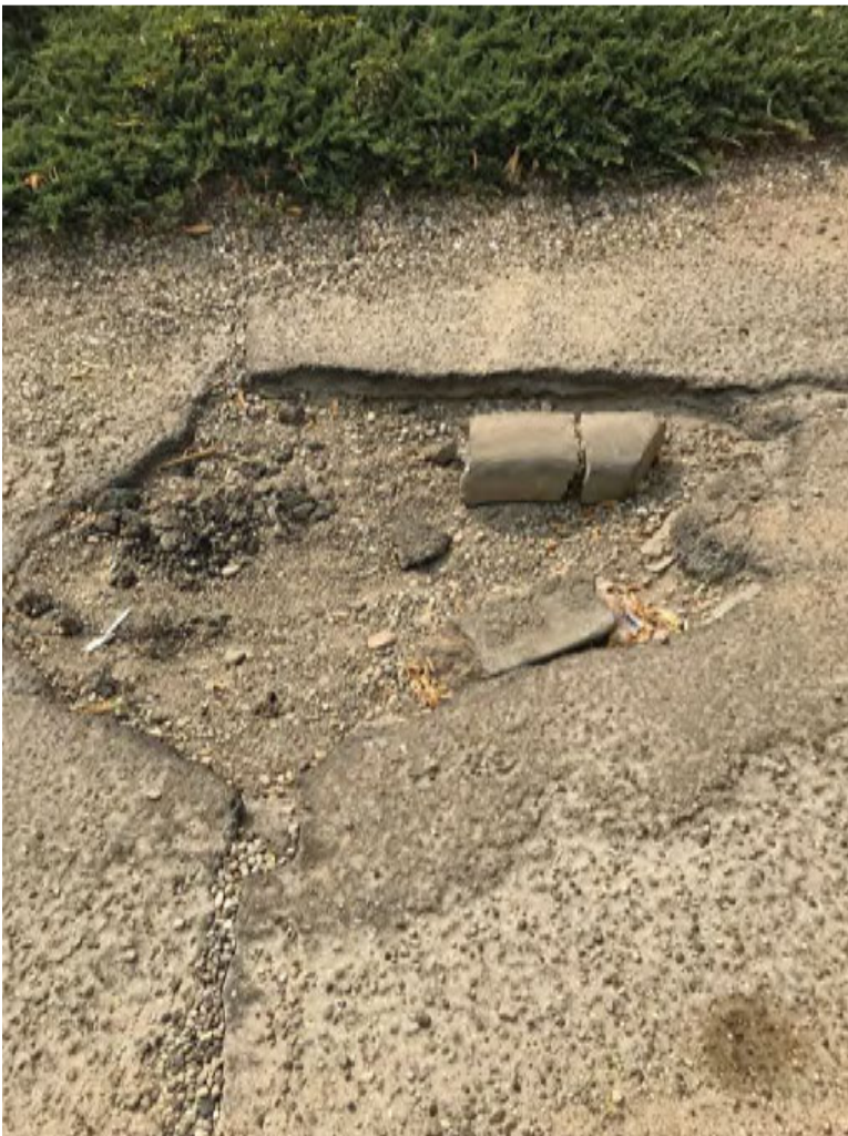
Large pothole in the alley behind DWF Wholesale Florist.
